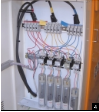
4 THE POWER FACTOR CORRECTION UNIT FITTED TO THE MAIN SWITCHBOARD HAS IMPROVED THE ZOO'S POWER FACTOR FROM 0.90 TO 0.99.
